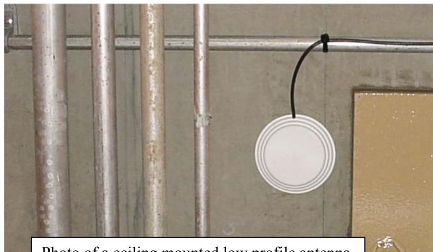
Photo of a ceiling mounted low profile antenna.
